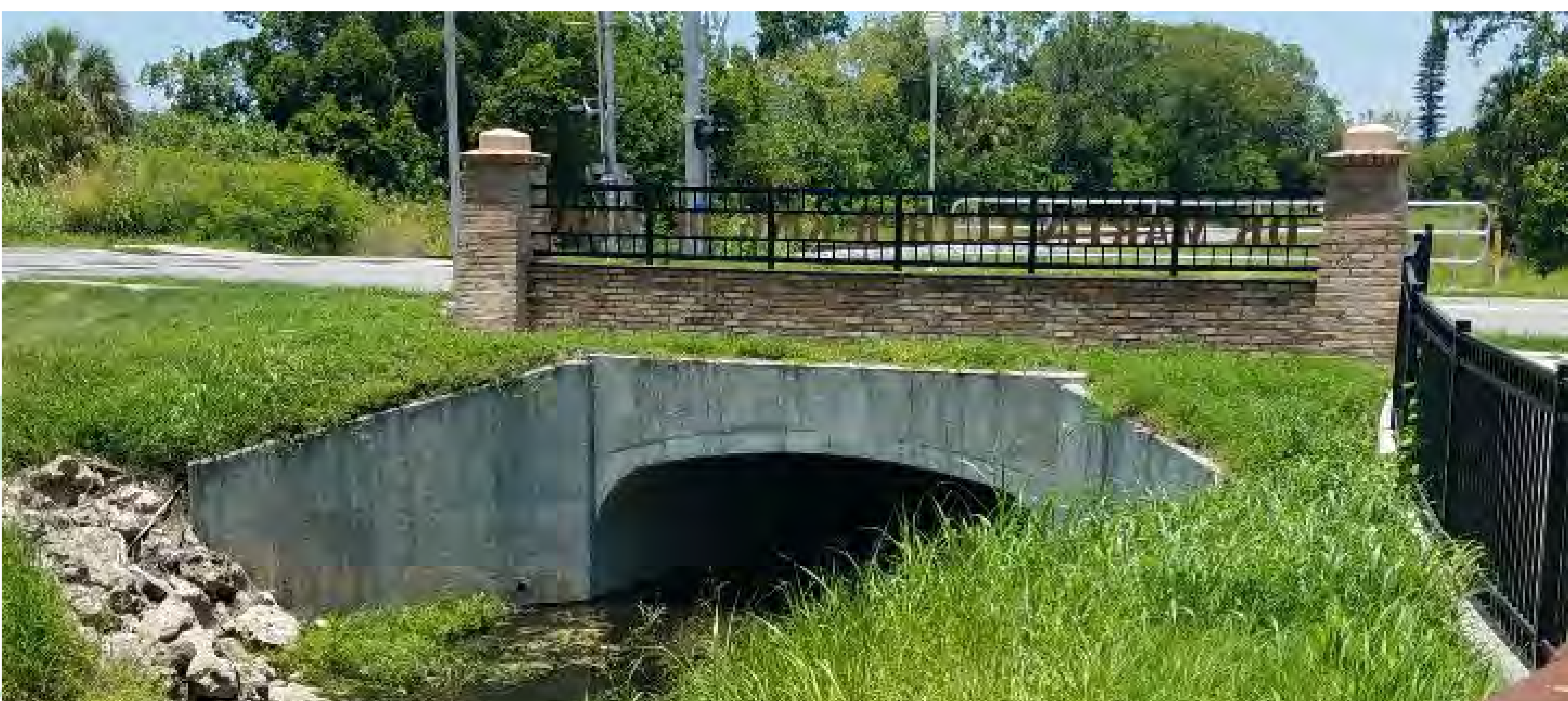
Box Culvert Bridge (North and South ends of Dr. Martin Luther King Jr. Trail)
