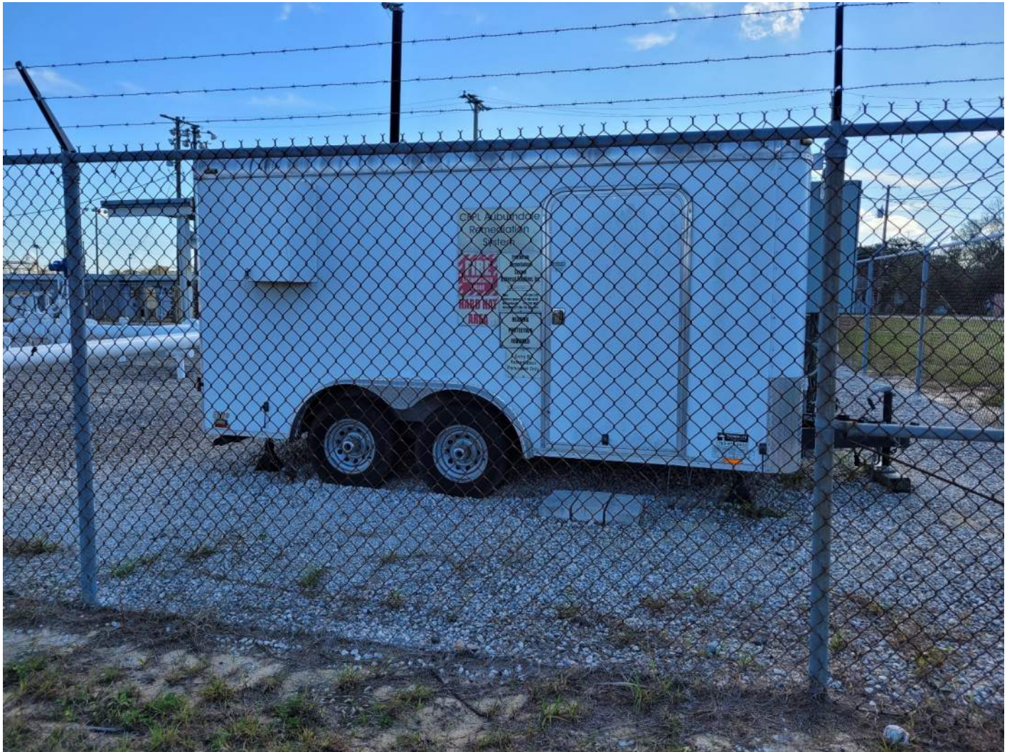
Map ID 6: Petroleum remediation system located on site
