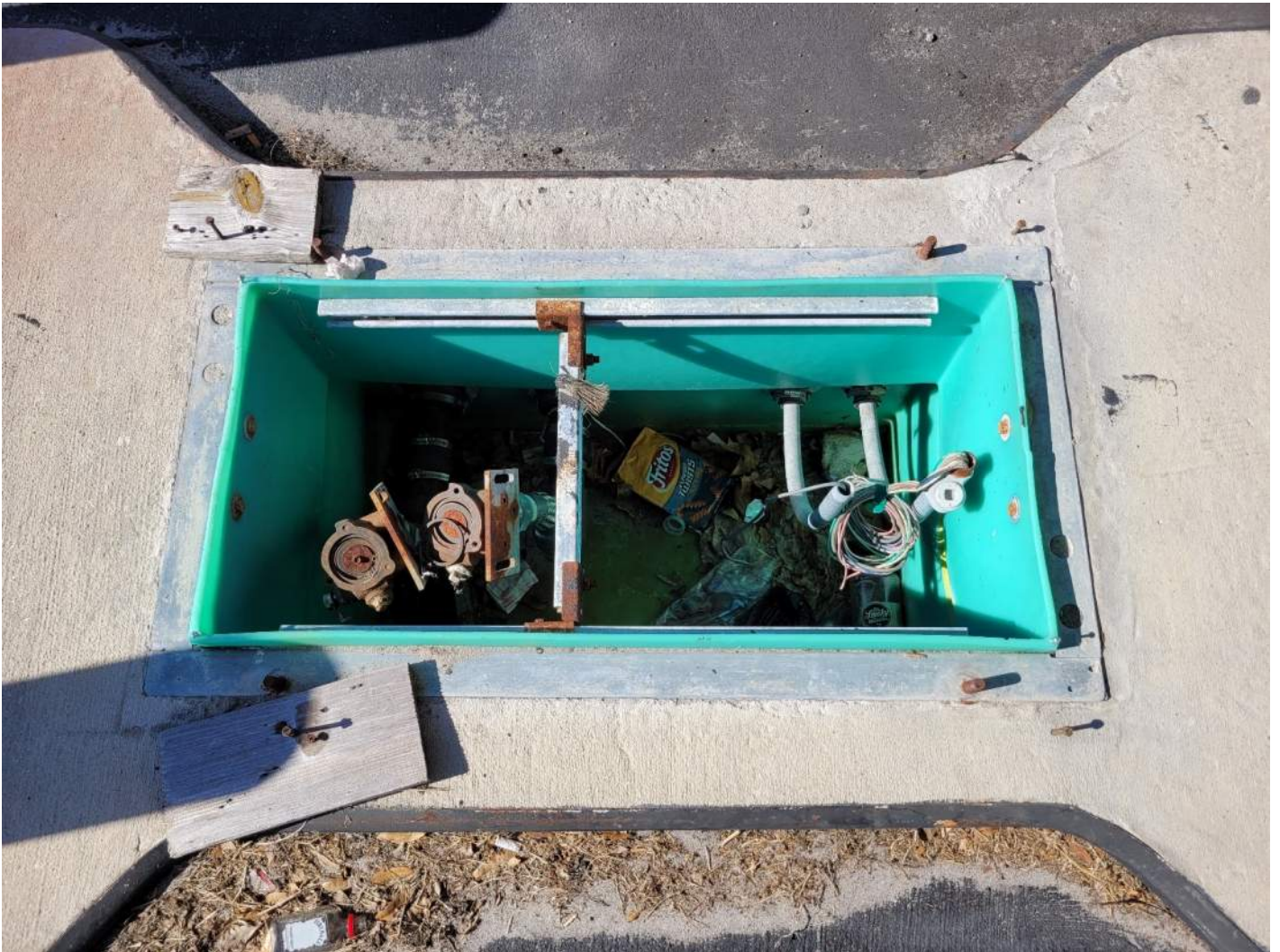
Map ID 4: Exposed internal piping observed at former dispenser locations
