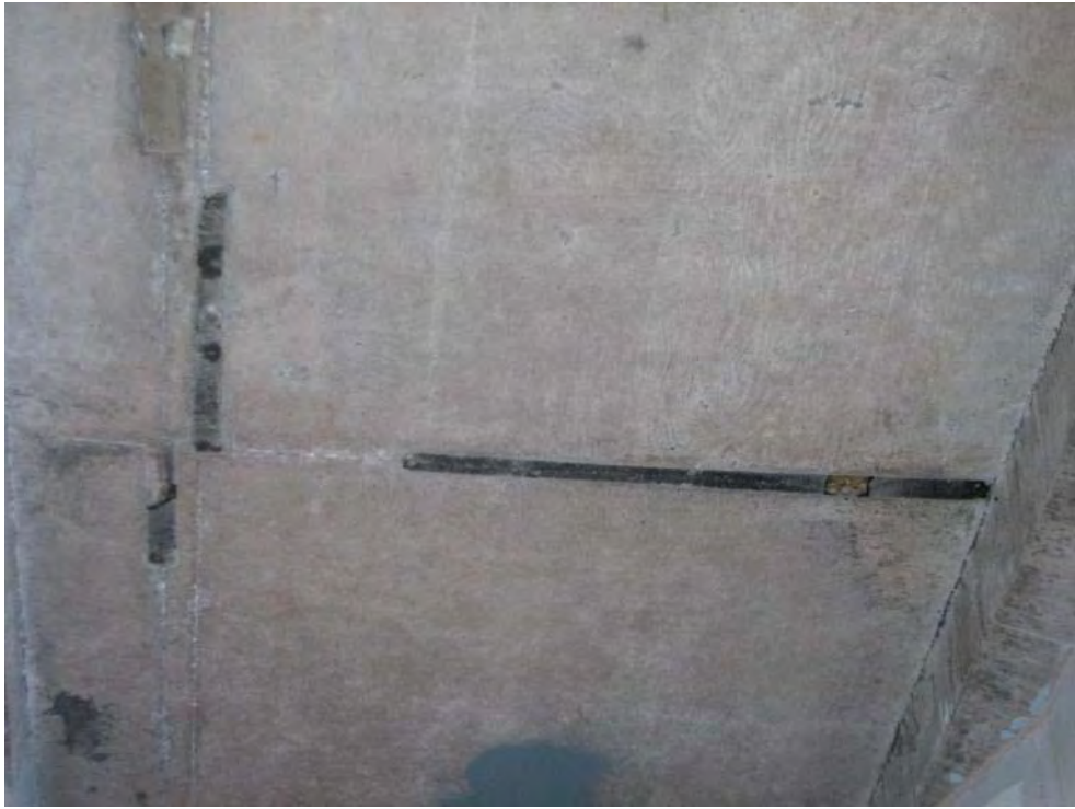
Homogeneous Material A – Residual tar paper
