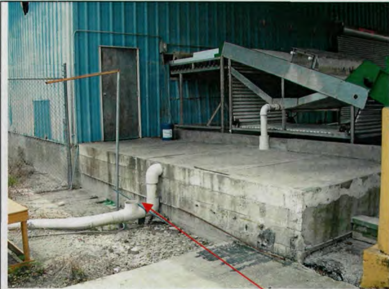
Discharge pipe from large washer. Note opening on top also
