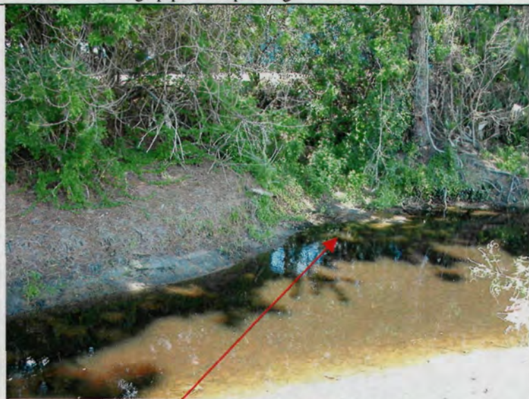
Outfall area near small vegetable washer. Note that the bank is widened and slope is eroded
