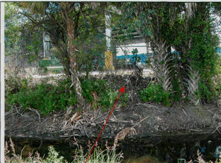
Unknown discharge pipe from packinghouse to the ditch.
