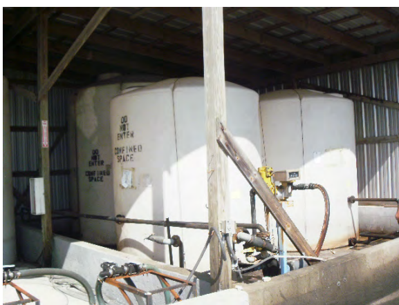
2010-9-9 TCI tanks in dike field not being used
