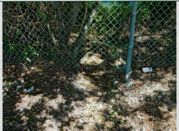
Hole cut in fence for possible discharge from small washer.
