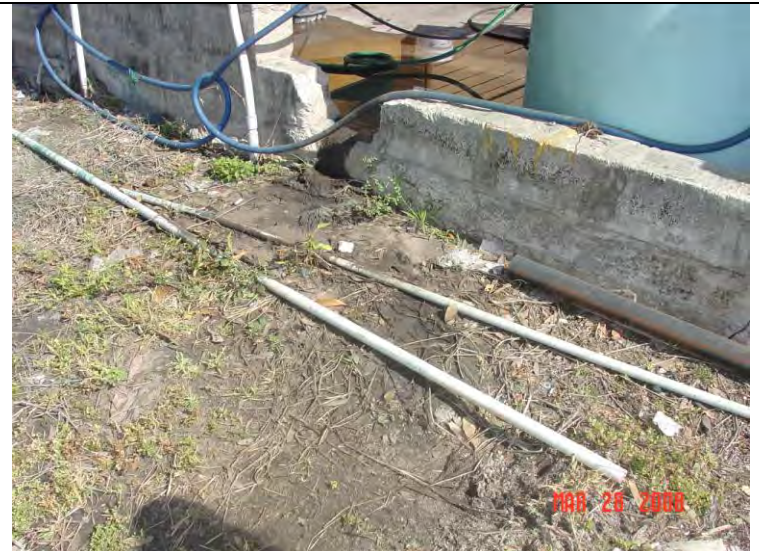
Photo 5 - Wash water discharge behind Wash Station
