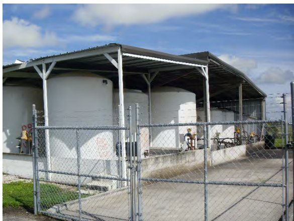
2010-9-9 TCI all tanks in 3 seperate dike fields
