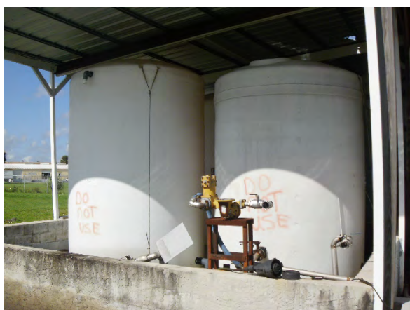
2010-9-9 TCI tanks in dike field
