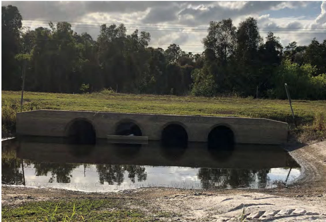
Photo 4. Cross drain on the east side of the roadway, photo taken during the dry season in March 2020.
