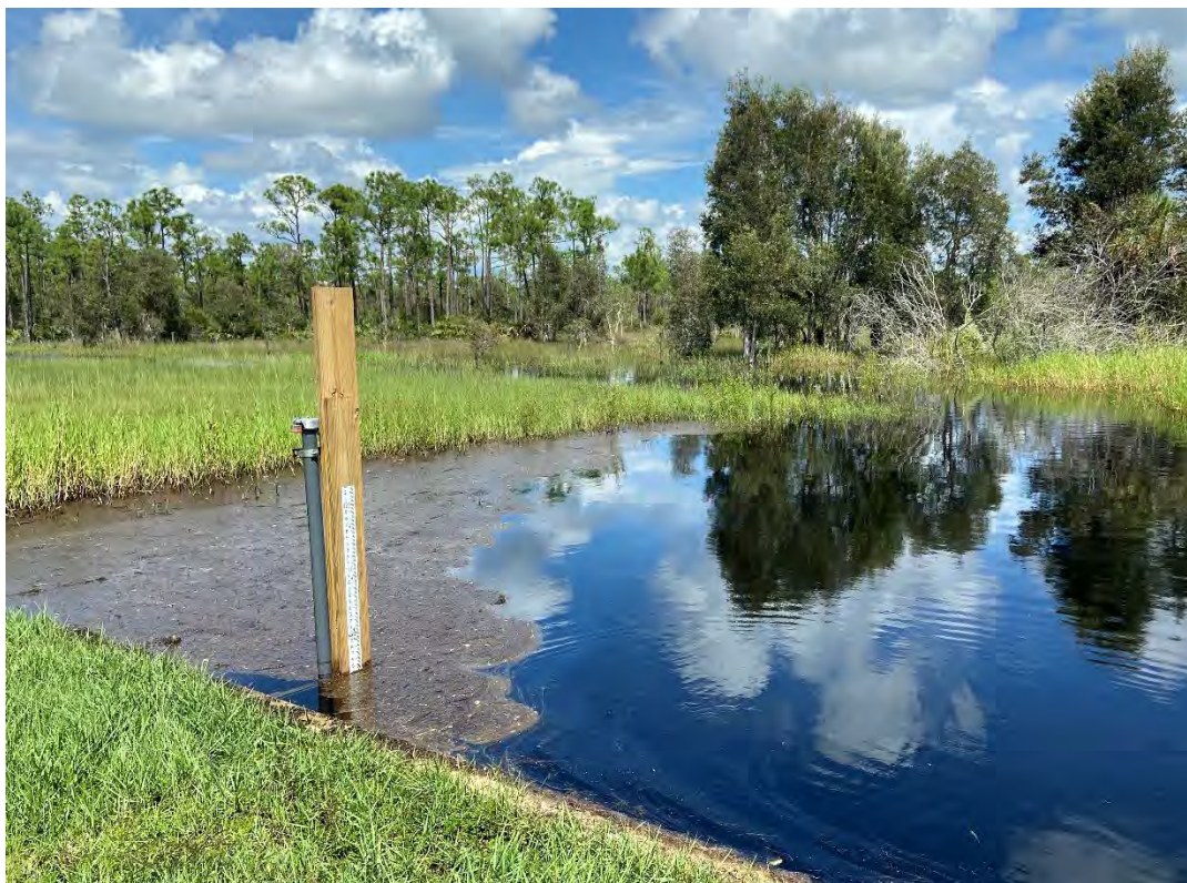
Photo 8. Cross drain with ditch in the background, photo taken during the wet season in September 2020.
