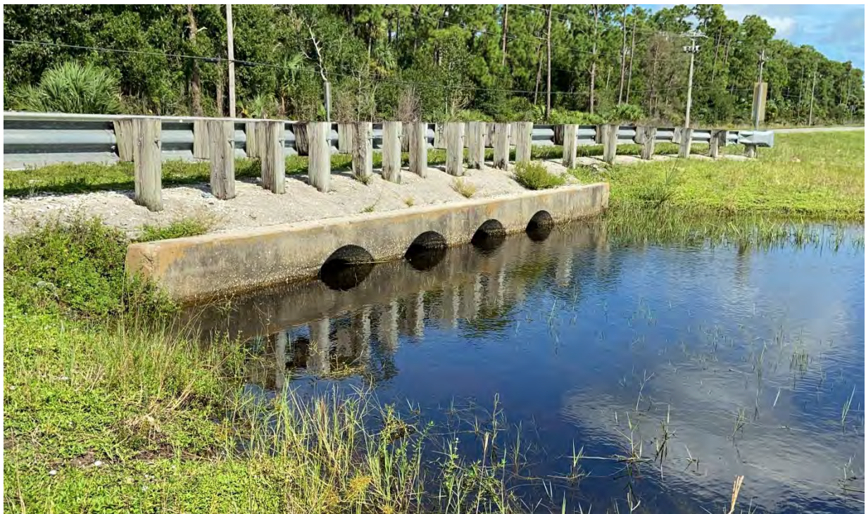
Photo 6. Cross drain on the east side of the roadway, photo taken during the wet season in September 2020.
