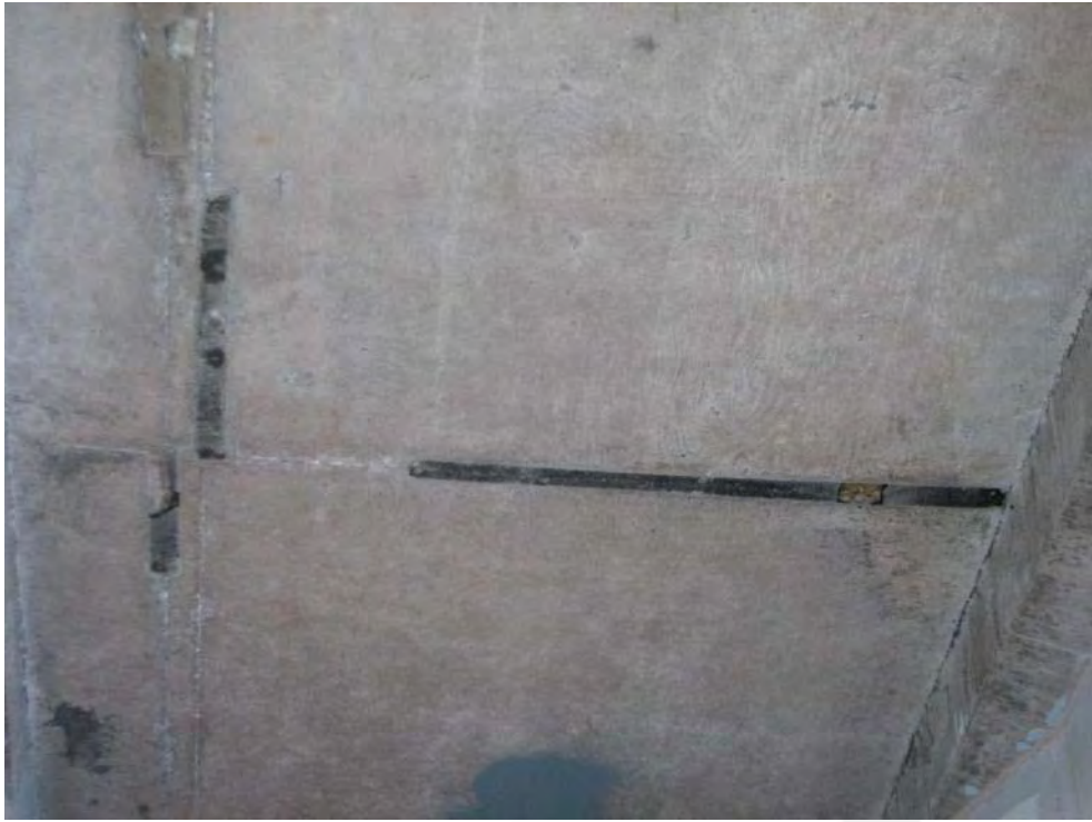
Homogeneous Material A – Residual tar paper
