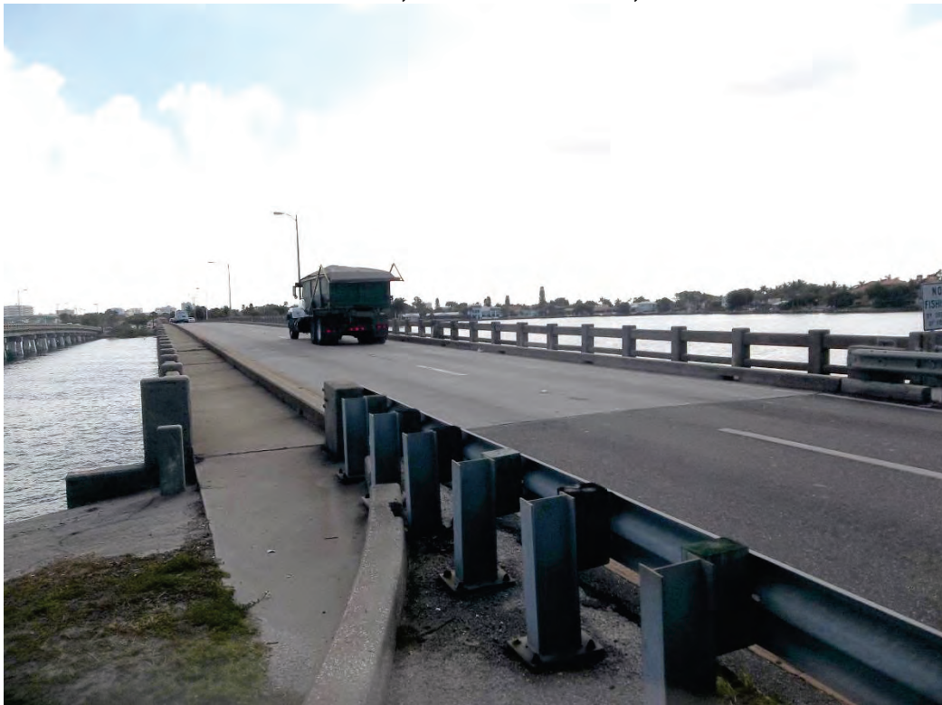
PHOTO 2 – 5/12/15 BRIDGE NO. 170951 – SR 789 OVER COON KEY WATERWAY – VIEW TOWARDS NORTHEAST SARASOTA, SARASOTA COUNTY, FL
