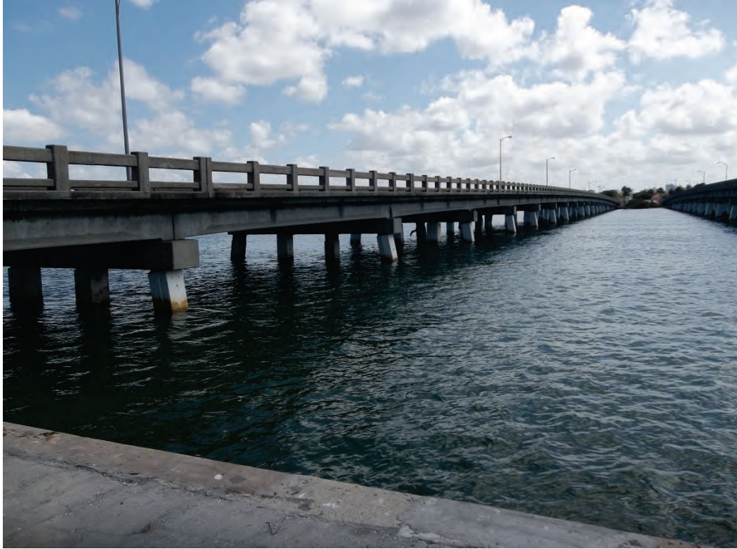
PHOTO 3 – 5/12/15 BRIDGE NO. 170022 – SR 789 OVER COON KEY WATERWAY – VIEW TOWARDS NORTHEAST SARASOTA, SARASOTA COUNTY, FL
