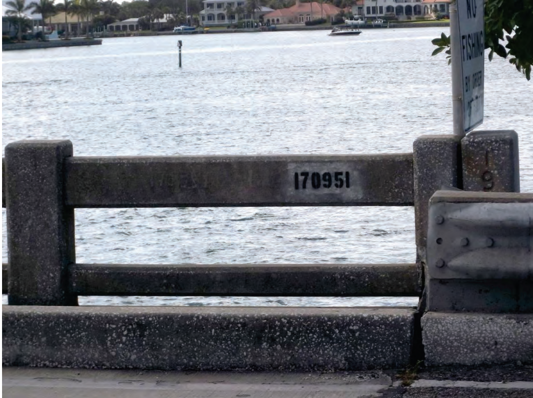
PHOTO 1 – 5/12/15 BRIDGE NO. 170951 – SR 789 OVER COON KEY WATERWAY – VIEW TOWARDS SOUTHEAST SARASOTA, SARASOTA COUNTY, FL
