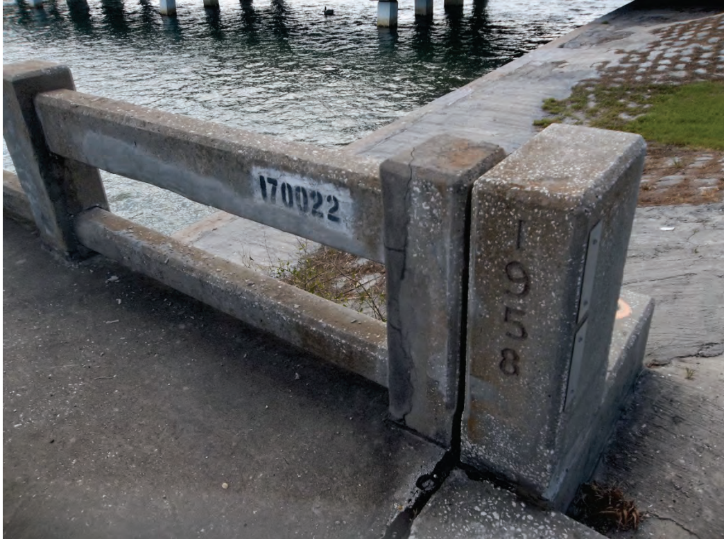
PHOTO 1 – 5/12/15 BRIDGE NO. 170022 – SR 789 OVER COON KEY WATERWAY – VIEW TOWARDS SOUTHEAST SARASOTA, SARASOTA COUNTY, FL
