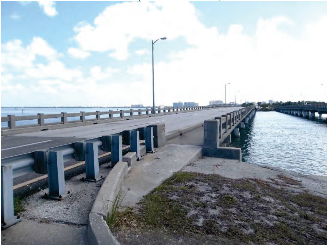
PHOTO 2 – 5/12/15 BRIDGE NO. 170022 – SR 789 OVER COON KEY WATERWAY – VIEW TOWARDS NORTHEAST SARASOTA, SARASOTA COUNTY, FL
