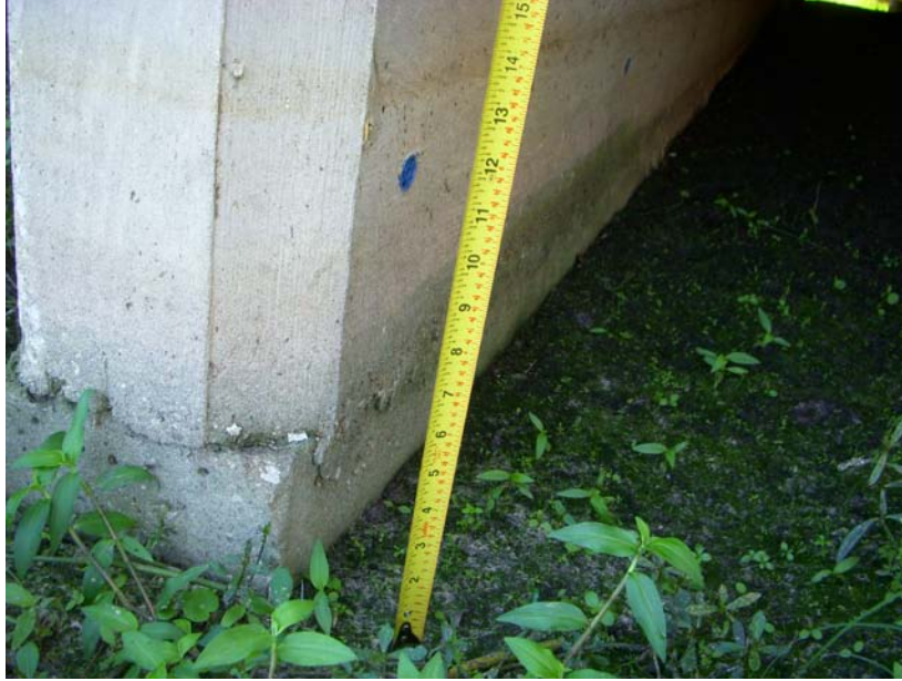
Stain Line Measurement
